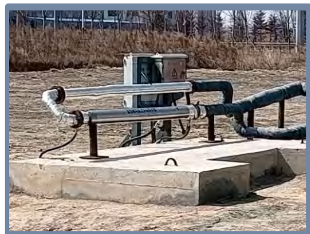
东辛采油厂(30kw)
